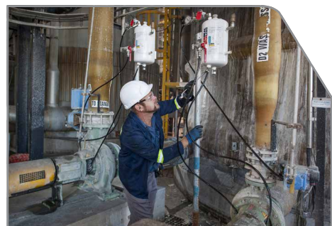
Continuous loop flushing and lubricating systems supplied by AESSEAL®, fitted to pumps at Mondi Richards Bay.
