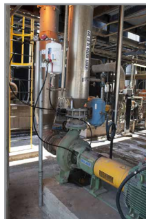
After: Pump and mechanical seal at Mondi Richards Bay, fitted with AESSEAL® continuous loop flushing and lubricating system.
